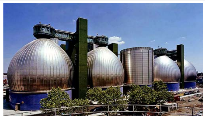
Figure 2: Photos of Newtown Creek WRRF egg shaped digesters.
